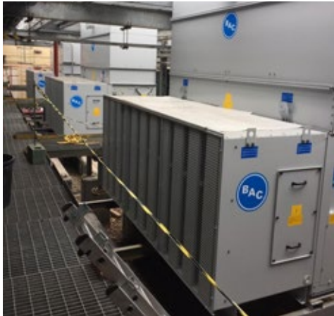
Intake Sound Attenuation
