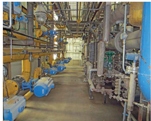
PSA plant with Jamesbury valves kept up to date (4 PSA vessels replaced in 1998).
