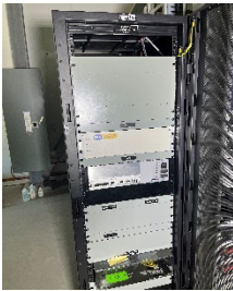
13) Open Air Insulated Station DIFF Relay Top Bus Panel 8W-1
